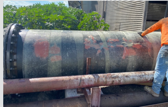
Figure 2 Repair putty was used to repair and seal leaks
