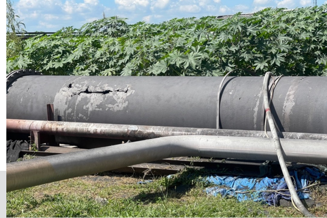
Figure 1 Severe degradation in critical cooling water pipe
